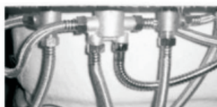
1 Cold/Hot Water Switch
